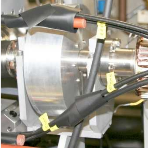
Figure 18: The connectors wrapped in black tape. In the background the housing of an ICT is visible.
