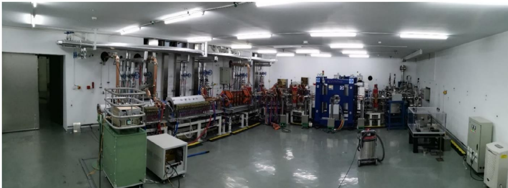
Figure 2: Photo of the accelerator and FEL oscillators in the semi-underground tunnel.
