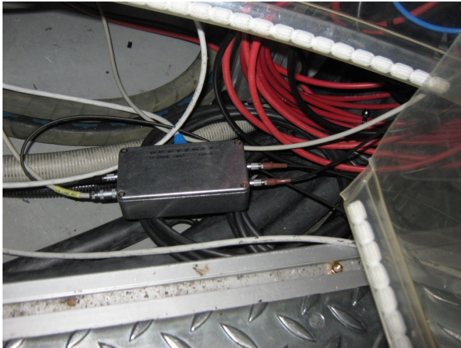
Amplifier in the tunnel
