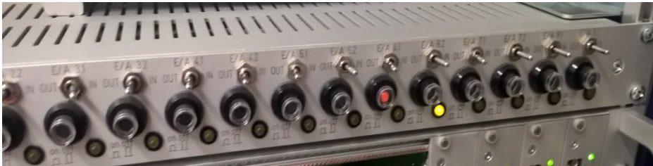
Power control unit – refer to the documentation attached on the rack for details
