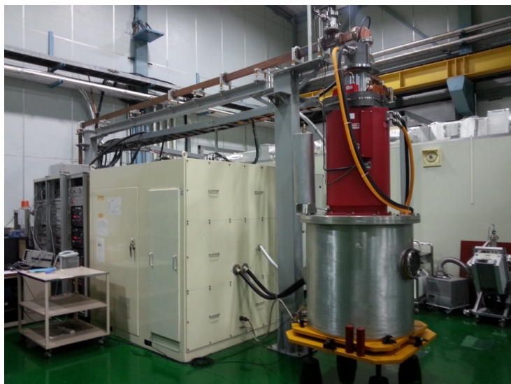
High power RF source for accelerator components
